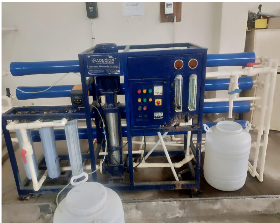
KBA MEN'S HOSTEL RO PLANT
