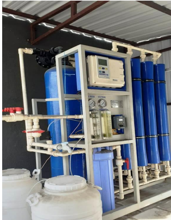
TBAK LADIES HOSTEL NEW BLOCK TERRACE RO PLANT
