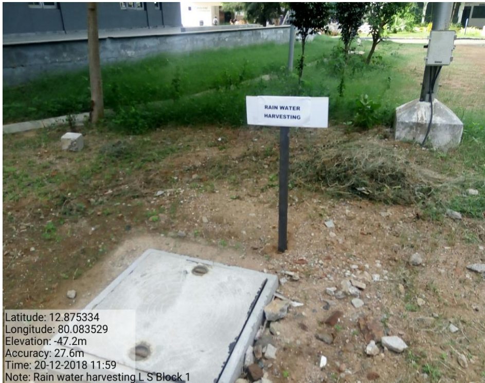
RAINWATER HARVESTING PIT AT LIFE SCIENCE BLOCK
