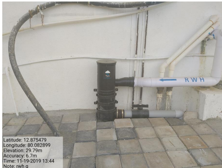
FILTER UNIT IN RAINWATER HARVESTING SYSTEM (ARCHITECTURAL BLOCK)
