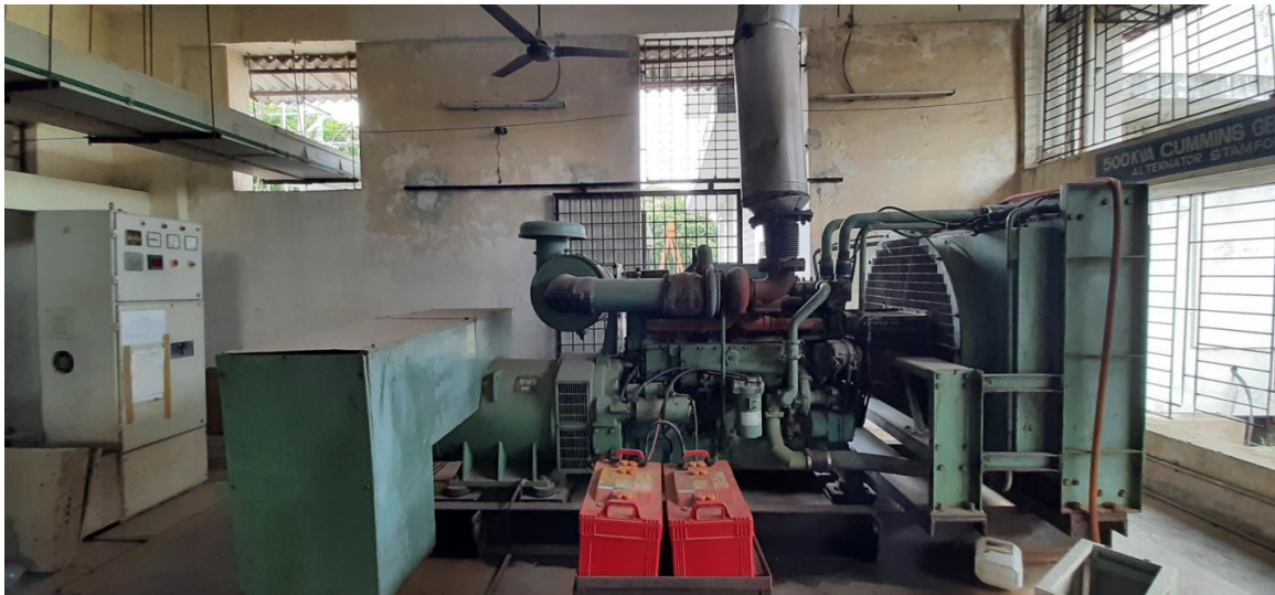
INDOOR DIESEL POWERED GENERATORS OF 500 KVA
