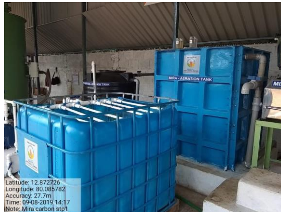
Mira carbon sewage treatment plant
