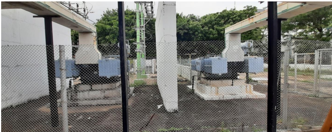
11 KV HT POWER SUPPLY / 8 00 KVA TRANSFORMERS
