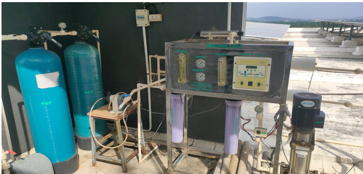
AERONAUTICAL BLOCK RO PLANT
