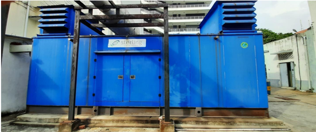
OUTDOOR DIESEL POWERED GENERATOR OF 750 KVA
