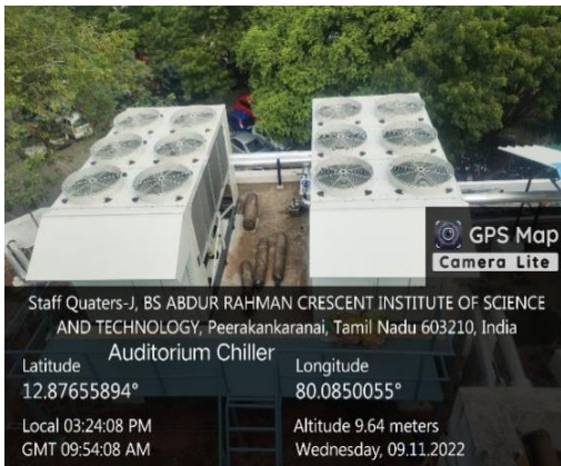
90TR capacity Auditorium Chillerplant
