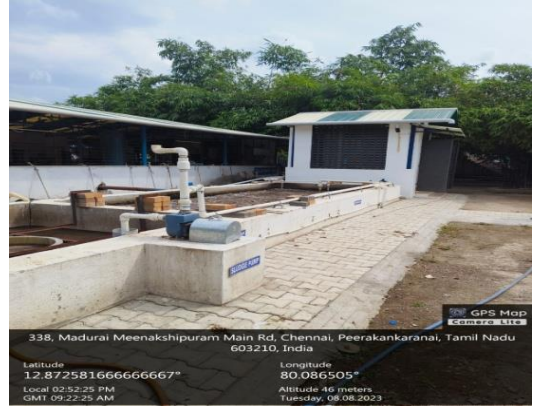
STP 100KLD capacity Increased in Men's Hostel
