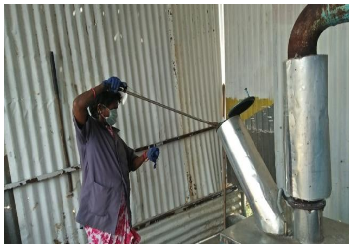
HANDLING OF INCINERATOR
