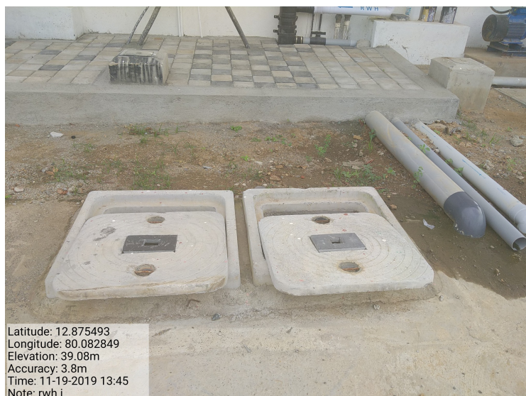
RAINWATER COLLECTION SUMP (ARCHITECTURAL BLOCK)
