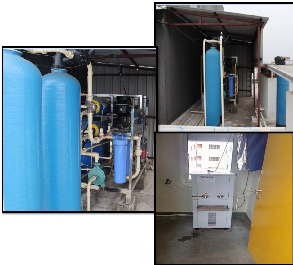
T. B.A.K Hostel, RO water facility
