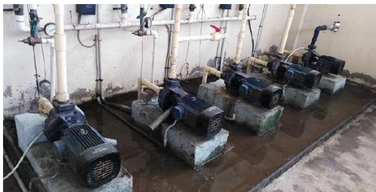
New hostel pumps
