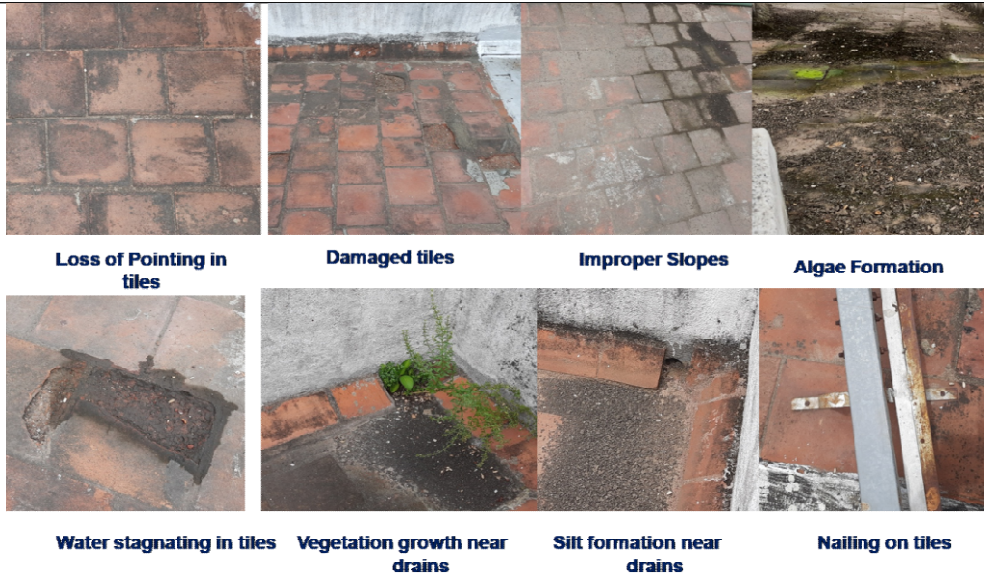
Figure 7: Anamolies in Clay tile finish
