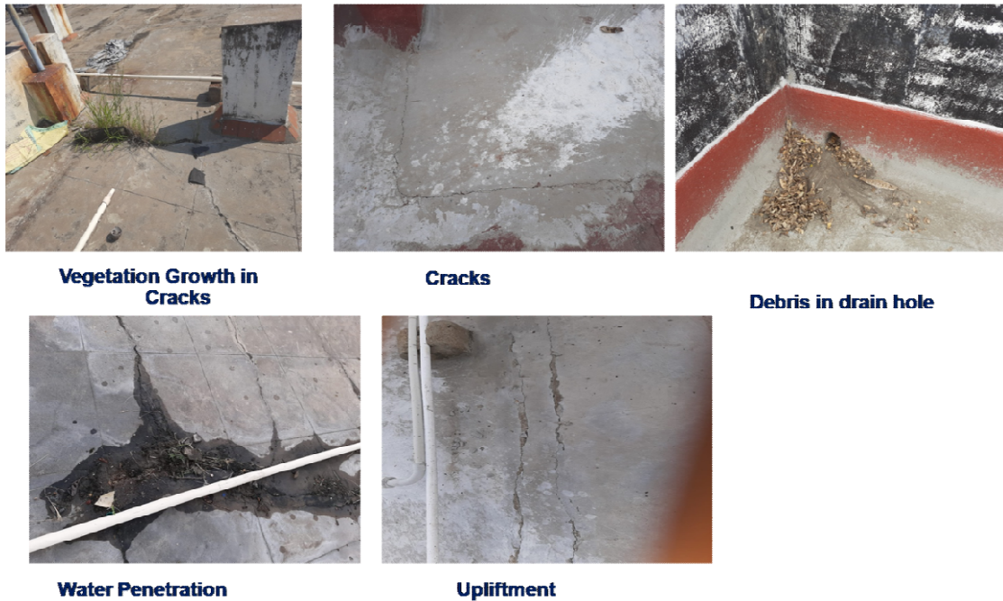
Figure 8: Anamolies in cement mortar finish
