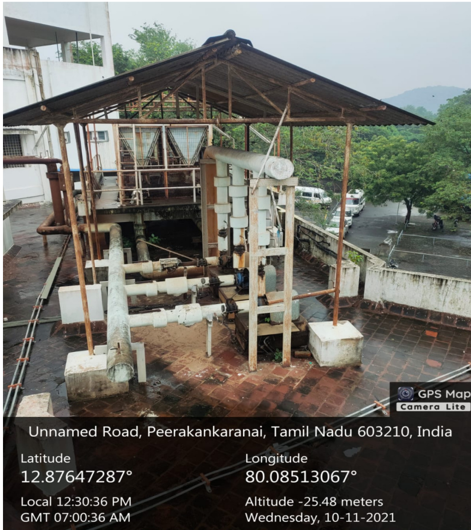
AIR-COOLED CHILLER PLANT
