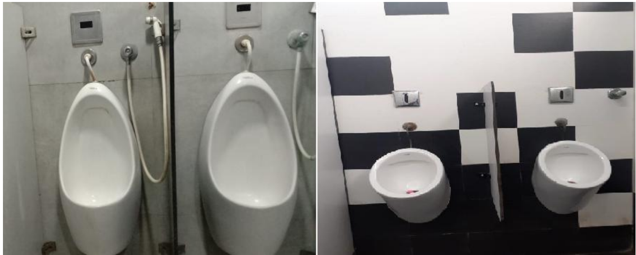
Urinals with automatic flush controller
