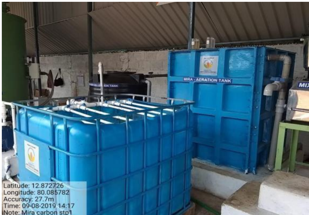
Mira carbon sewage treatment plant
