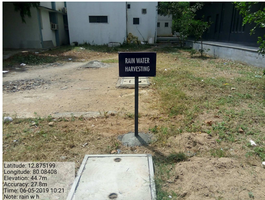
RAINWATER HARVESTING PIT
